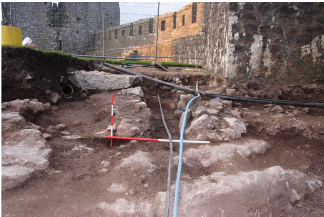
Photo 9: Overview of northern end of site showing the fall of the natural bedrock in the foreground, with structure (132) behind, remnant concrete slab for retaining wall to rear left and extensive truncation from modern services, scales 1m and 0.5m.
