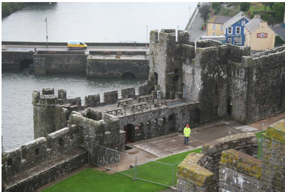
Photo 1: View of St. Anne's Bastion taken from the Keep, view east, prior to groundworks.
