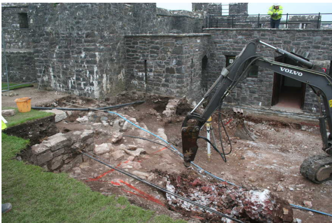
Photo 12: Machine excavation of bedrock to form the footprint of the new café, with red spray-paint line showing agreed limits of groundworks to preserve archaeological remains.
