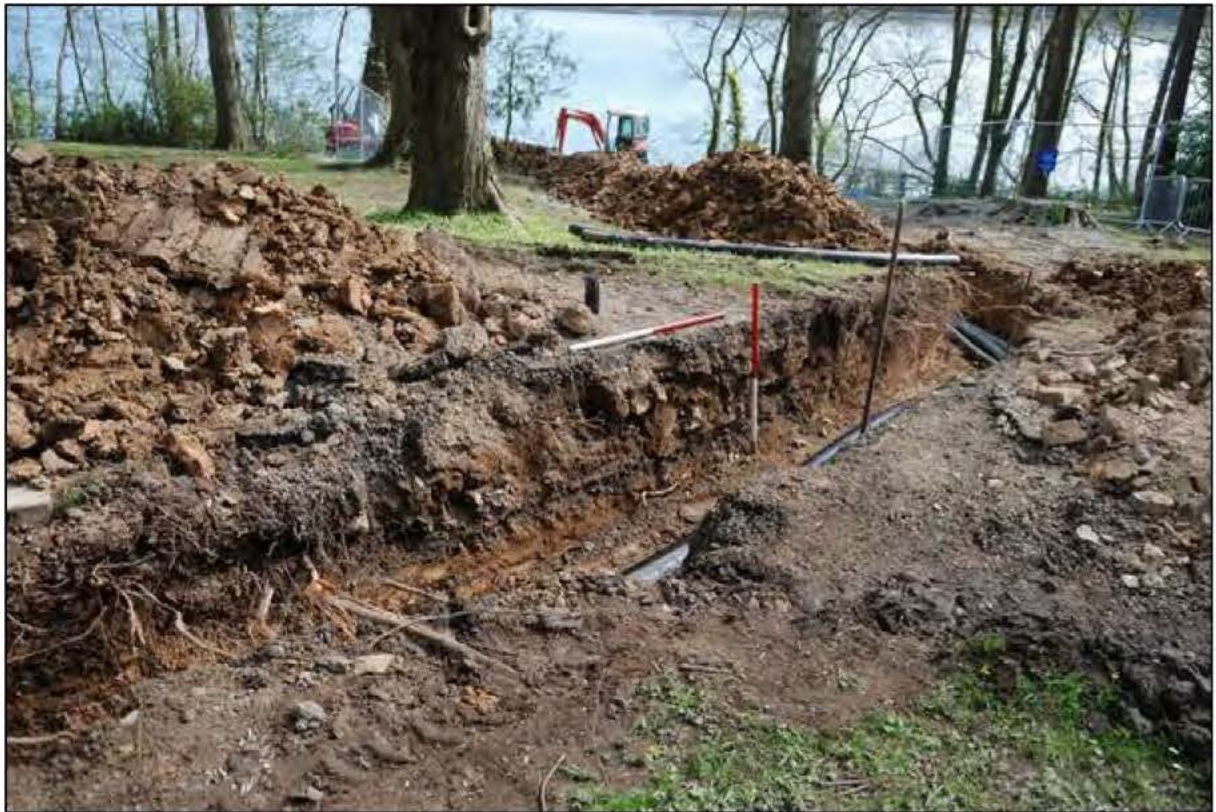
Plate 13: Deposits below the path to the rhododendron walk
