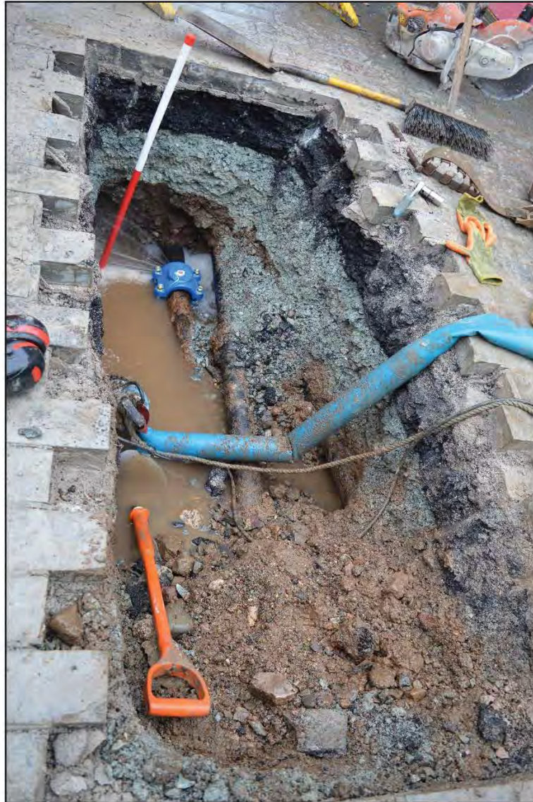
2. Trench following completion of excavation, showing identified leak (scale 1m, view from the North-Northeast)
