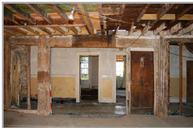
Plate 40: Ground floor aisle truss in hall. The upper central horizontal beam dated c. 1620
