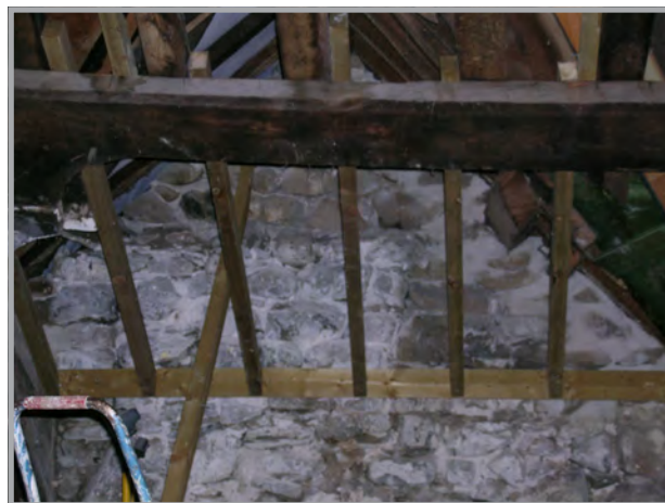
Plate 33: The discolouration co-incides with straight joints in the masonry which could indicate blocking or an earlier structure
