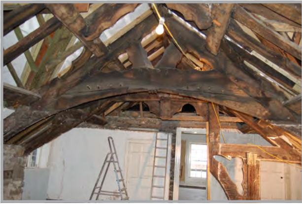
Plate 23: The aisle truss before renovation can be seen behind the collar-beam truss. The south aisle post is missing
