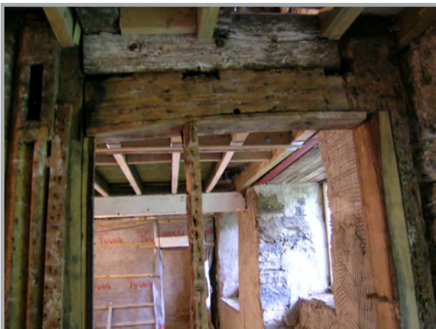
Plate 43: Mortise in aisle truss and notches for joists on the cross-passage side
