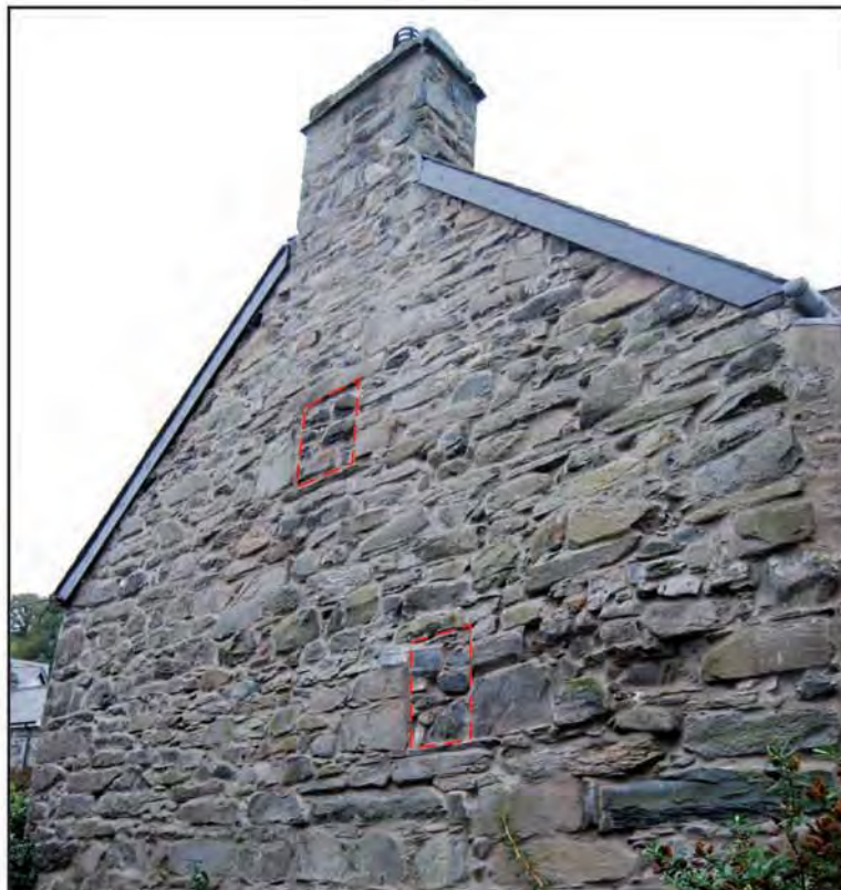
Plate 1: South-west facing image of north facing gable showing two blocked windows
