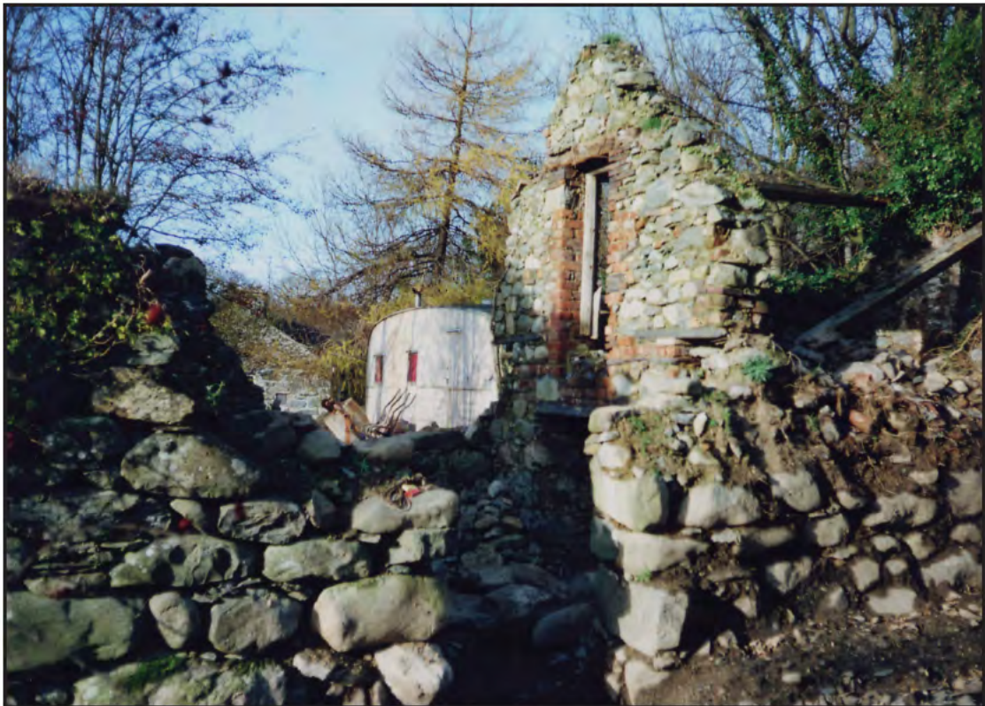
Plate 2. West facing image of the middle gable prior to collapse.
