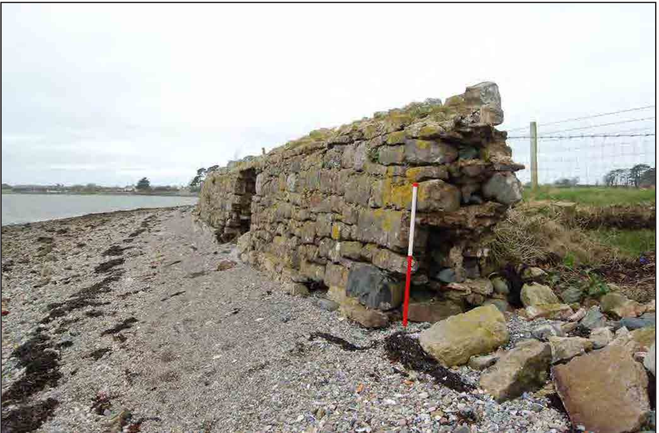
Plate 21: Collapsed/breached sea defence wall at Brynsiencyn
