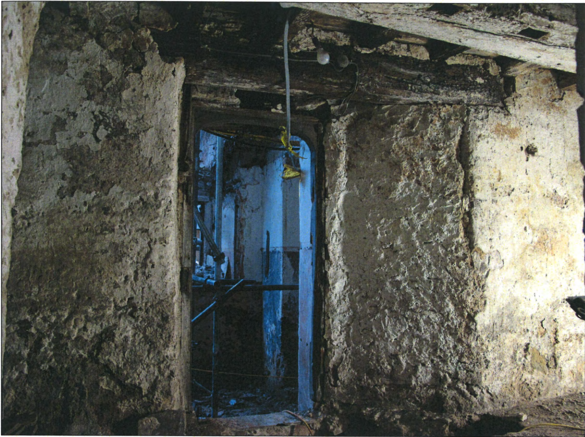
Blocked door and lintel at entrance to sixteenth century cellar, victorian corridor beyond.
