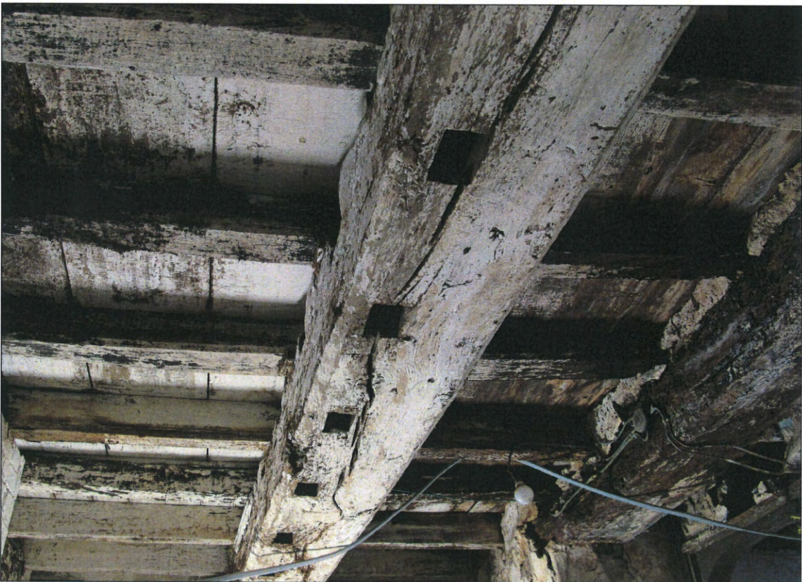
Re-used beam in cellar with sockets for joists and sockets for stud panelling.
