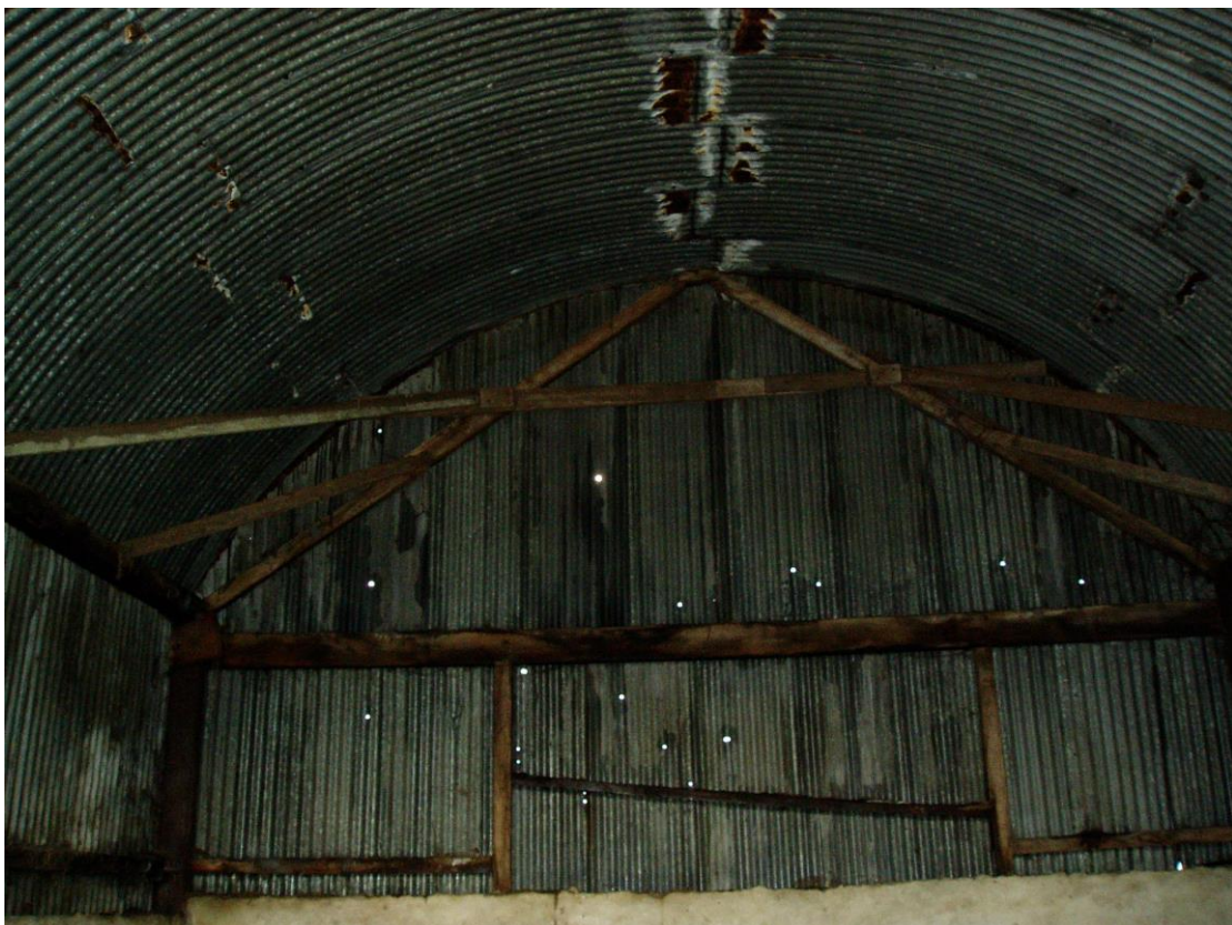
27) Interior of Building A Looking South West Showing Crane Arrangement
