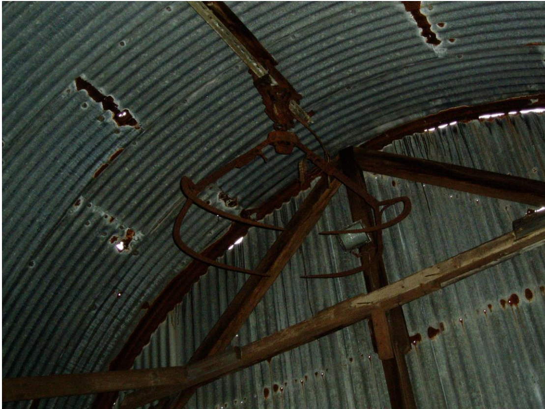
50) Interior of Roof D Showing Crane Equipment
