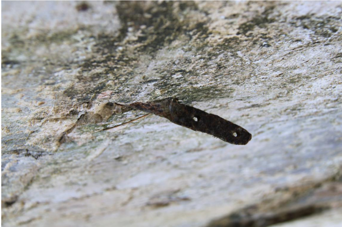
Plate 27 - AD010-BR-027 - Misc metal bracket, internal, north wall.
