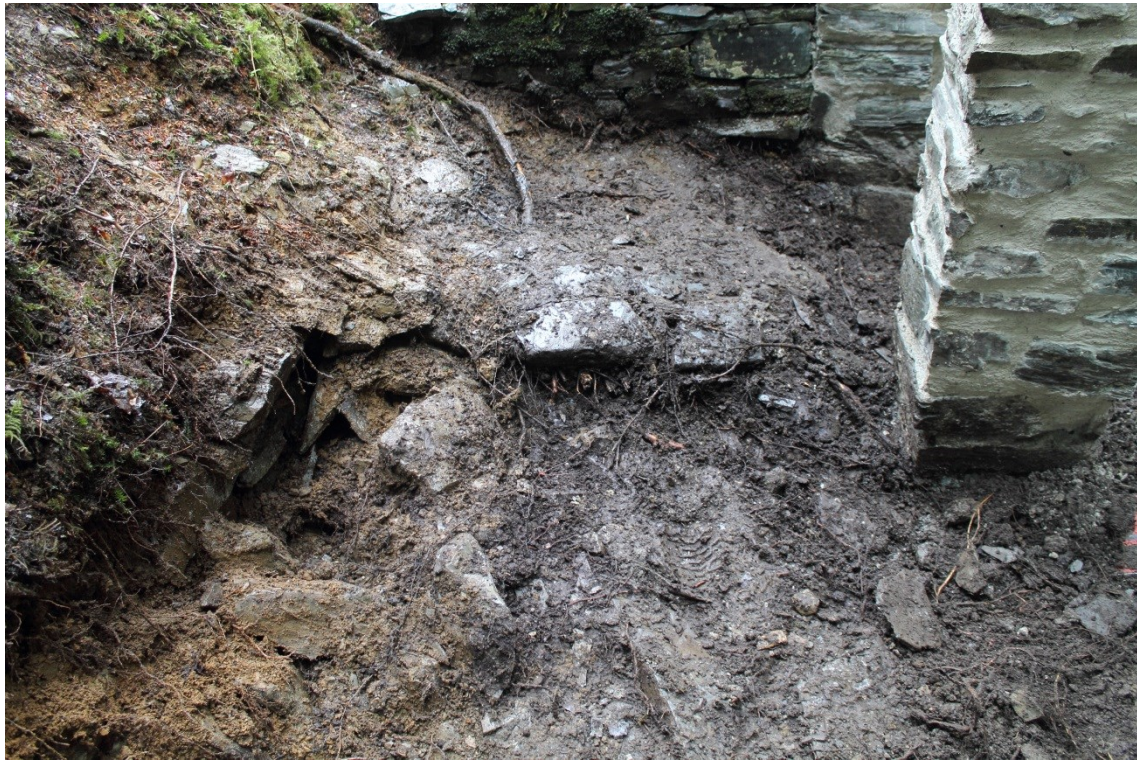
Photo 4: The loose dark silty soil lying above the collapsed stone of the retaining wall – looking northwest.
